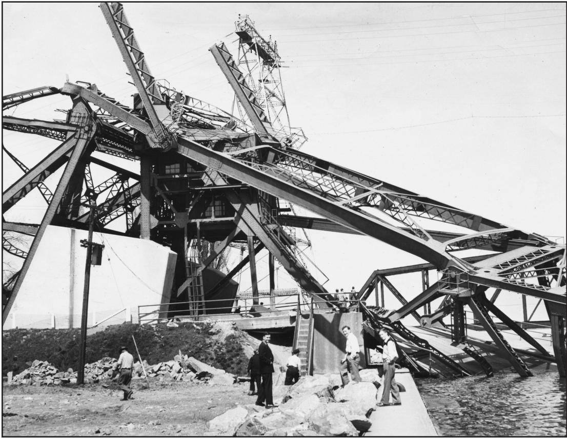
• Spectators get a close-up view of the damaged bascule bridge.
